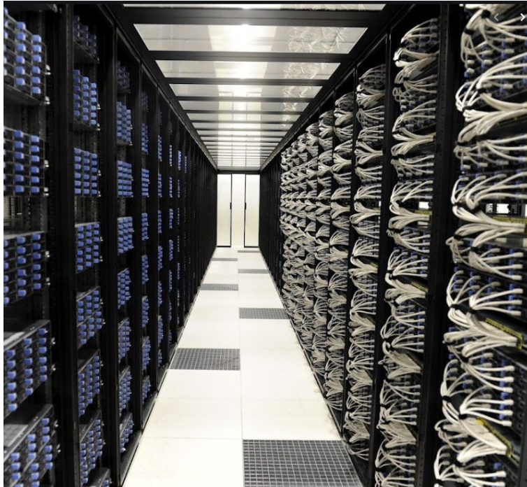
Figure 1.2: Data center with optical interconnects [7].
